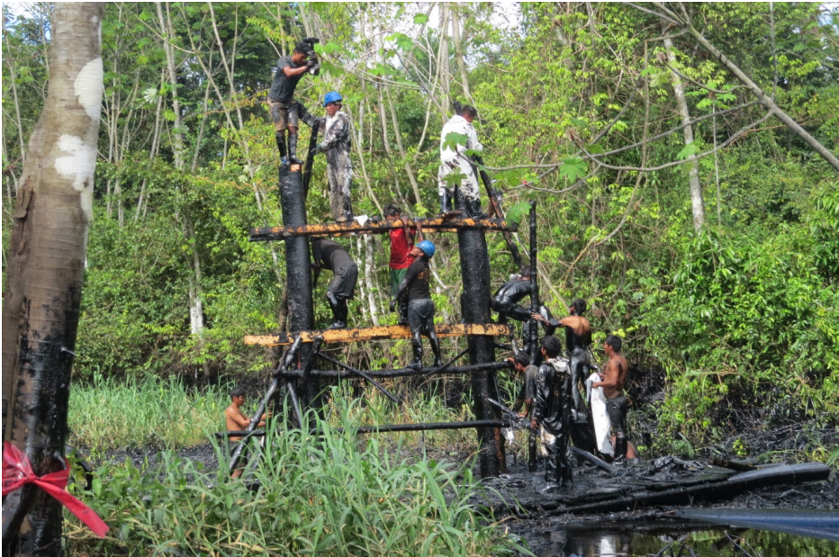
Photo 3: Cuninico residents inserting removing one of the wooden timber frames the supports the North Peruvian pipeline. The absence of heavy lifting equipment and limited white protective overalls are clearly visible (Photo given to me by a Cuninico resident who himself received it from a Petroperu worker and used with their permission, June 2014).
